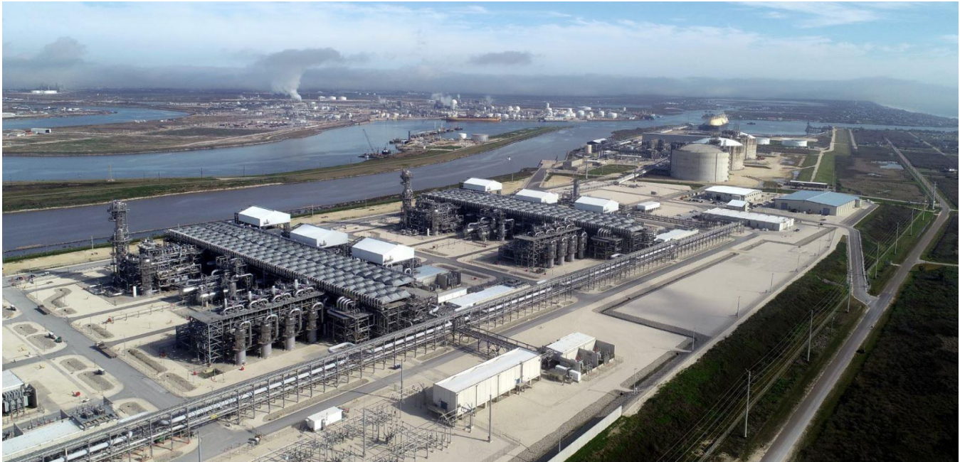
Figure 4. Freeport LNG – 2 of 3 Liquefaction Trains (Source: Freeport LNG Development, L.P.)
